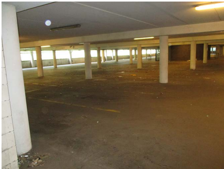
Photo 8. View of basement parking underlying all three towers of the office building.
